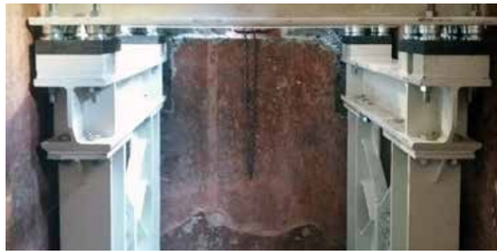
Contec separated the new vibrating system from the machine frame by installing it on a heavy-duty support construction
